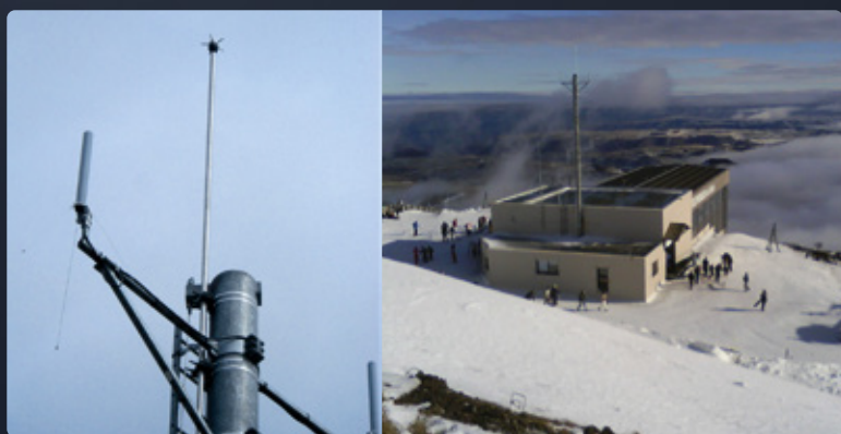
ESE air terminal in extreme climatic conditions
